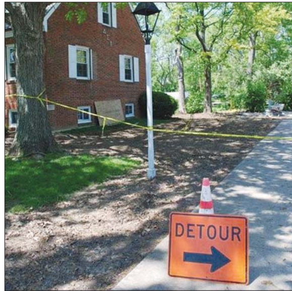
Central Office renovations have kicked into high gear! See full coverage beginning on page 37 of this issue.
